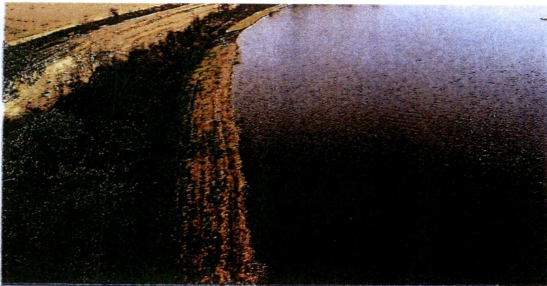
Photo 2. Helena WWTP South Wall Cell 3 Showing whole top of levee is gone
